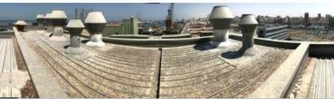
This roof has a Small Valley Gutter and an Eave Gutter at the far end of the roof and 1 downspout in each gutter. The gutter length is around 4.45 Meters. However, there is too much Bird Waste on the roof and in the gutters resulting in complete clogging of the drains and water then penetrates from the sheet terminations underneath the sheet and the gutter. Heavy Maintenance is required of this area as well as to replace the gutters since these are also rusted.
